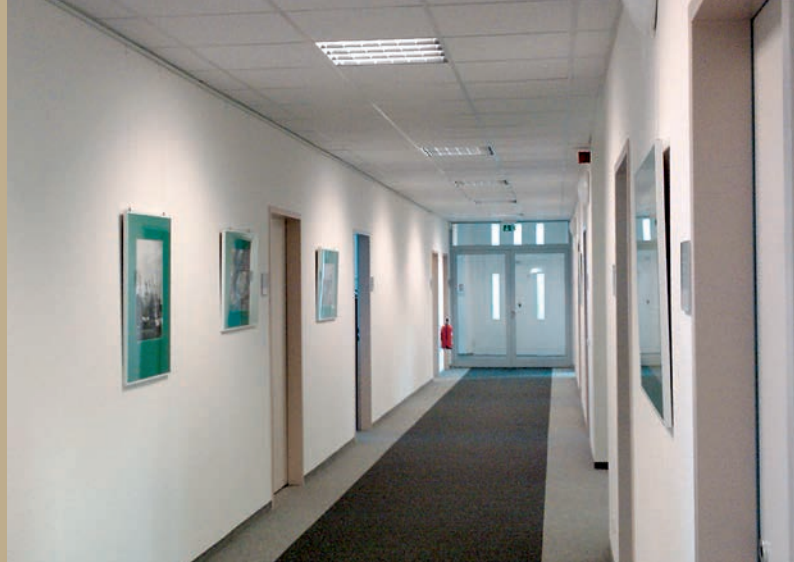
LED lighting on the third floor of an Institute building
